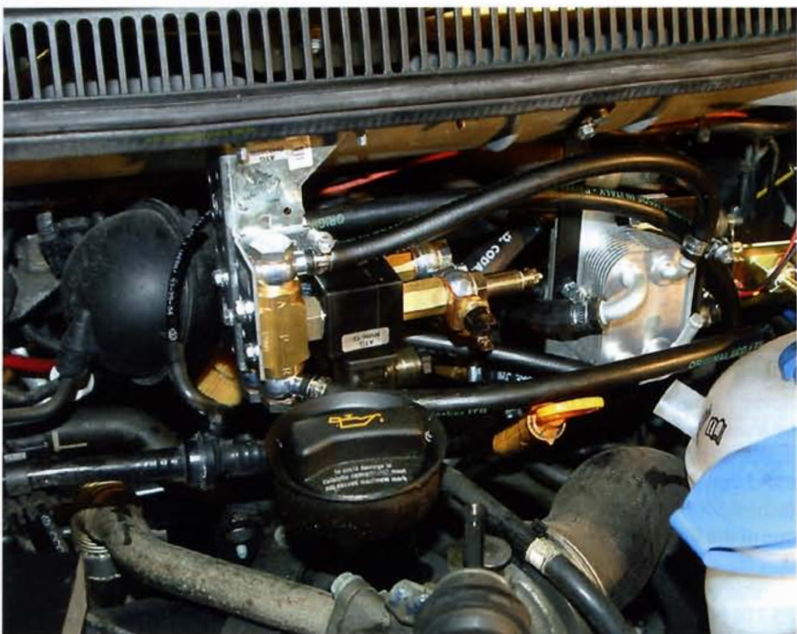
The heat exchangers and supplementary pump (the T5's own lift pump isn't suitable to pump vegetable oil) were fitted to the bulkhead. Mounting brackets are made to suit your own installation. Solenoid switches are also mounted on the underside of the rain channel.
